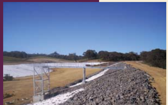
DUX® 300c at Daylesford WWTP
