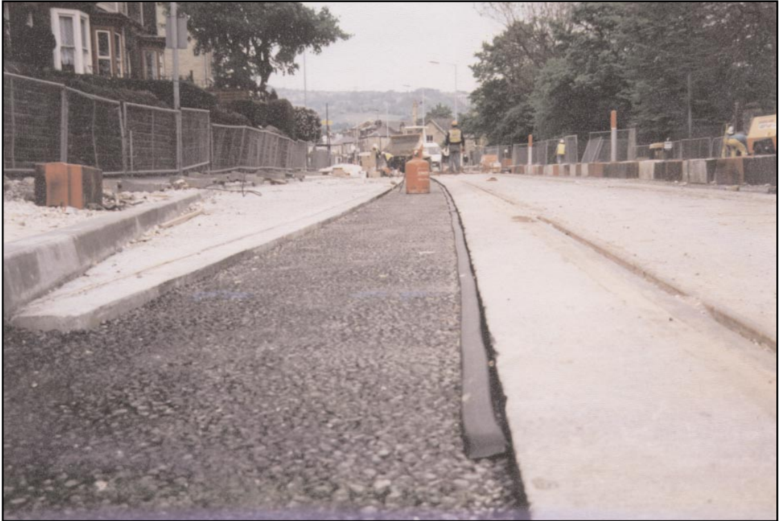
1. Densoband laid out against primed vertical surface of concrete tram rail bed prior to application.
