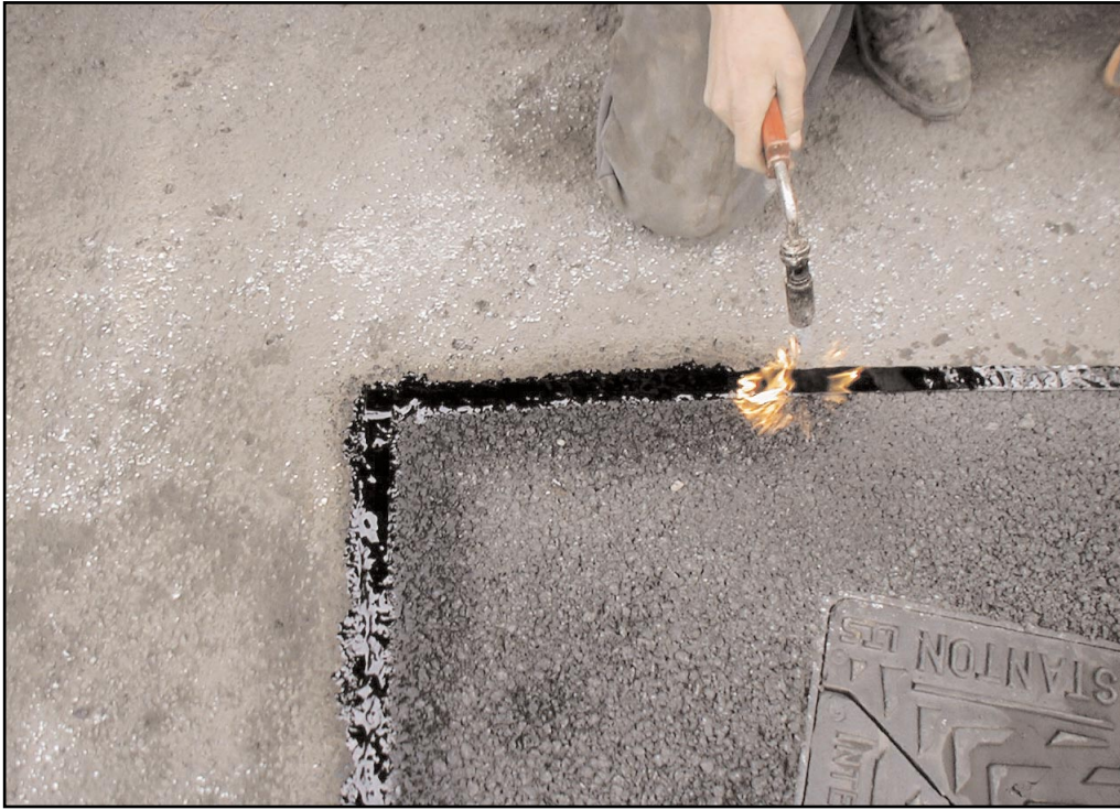
3. A gas flame is quickly passed over the Denso Overbanding Tape to fuse it into the joint surface.
