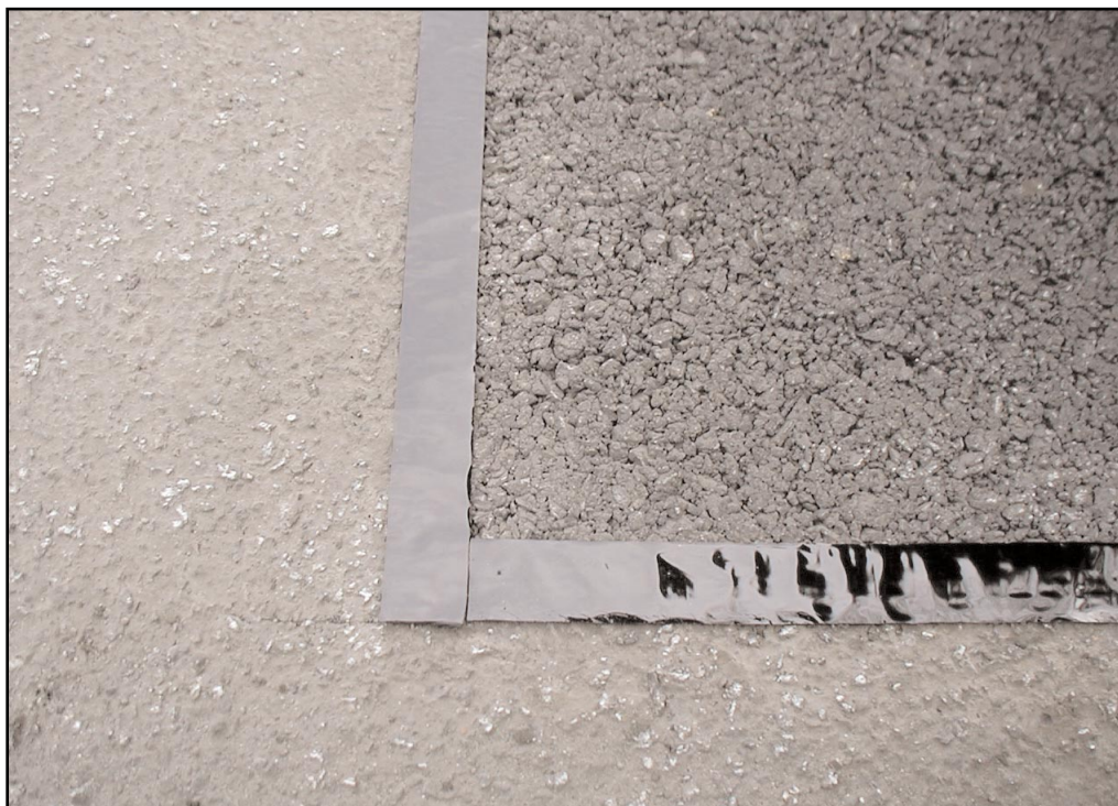
2. Denso Overbanding Tape is positioned over the joint between the new asphalt reinstatement and the existing road wearing course.
