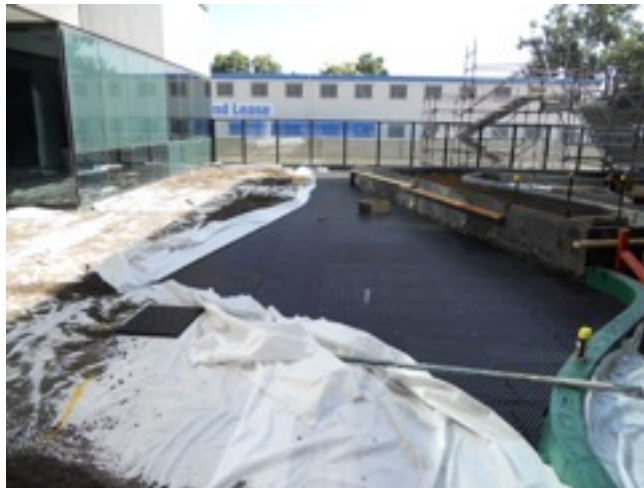
Royal Childrens Hospital 2011 NERO 30mm Drainage Cell & DUX 23c geotextile Contractor: Australian Native Landscape Constructions
