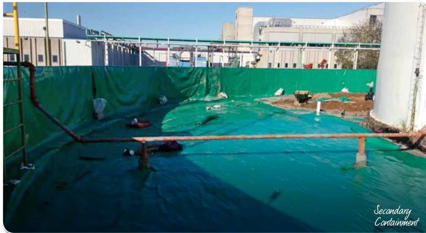
Biodigesters and Floating Covers
