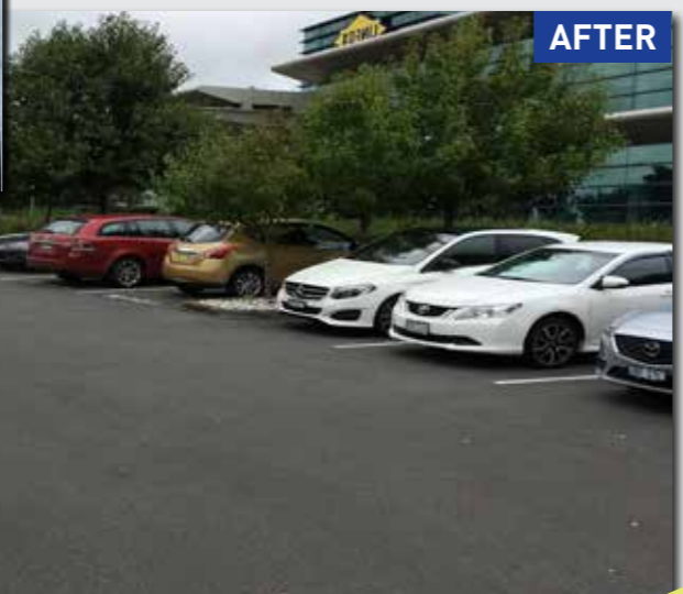
Installed in 2009, the pavement is in excellent condition in 2018. Linfox H/O, 56 English Street, Essendon Fields
