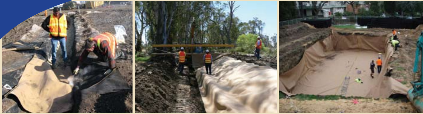
Seaming CANAL® at Bunnings with hot melt glue; Rolling out CANAL® at Gunbower Creek with laydown frame; Seamed CANAL® installed at Loreto College.
