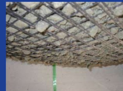
Effective separation using Fornit
